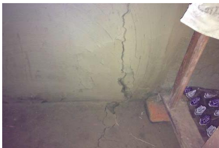
Photograph 2 : Elderly couple's hut having fissure due to ER earth work
